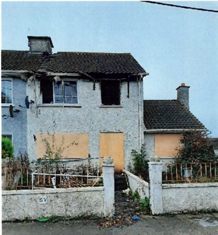
Photograph taken 1 st October, 2025
